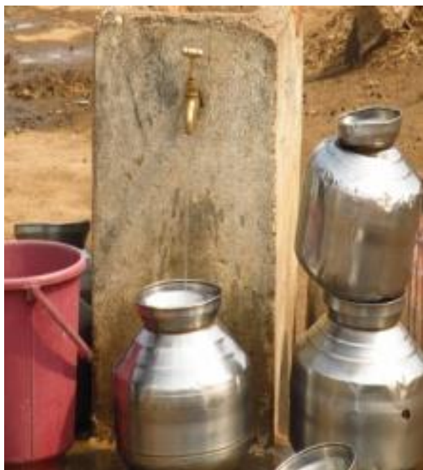
Water supply tap stand
