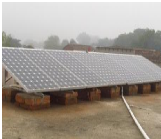
Solar panels supplying power for pumping
